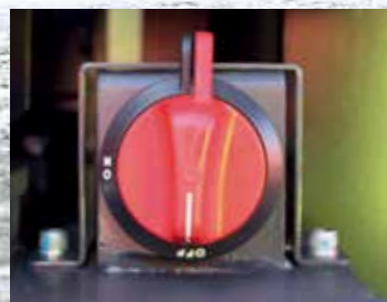
Battery cut-off switch
